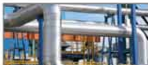
Pan Gulf Piping Solutions Complete Piping Systems
