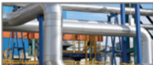
Pan Gulf Piping Solutions Complete Piping Systems
